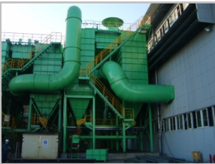
• Air pollution control equipments
