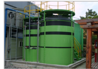
• Wastewater Treatment Facility
