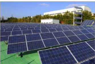
• Photovoltaic power generator in Eumseong Factory
